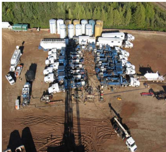
Frac equipment—aerial picture from the Nabors Rig #86 derrick on the O-76 well pad
