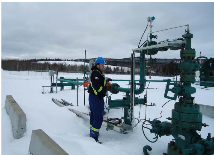
Instrument Technician Steve Evans conducting a well site inspection of the safety equipment on the D-48 well located on the D-48 well pad.
