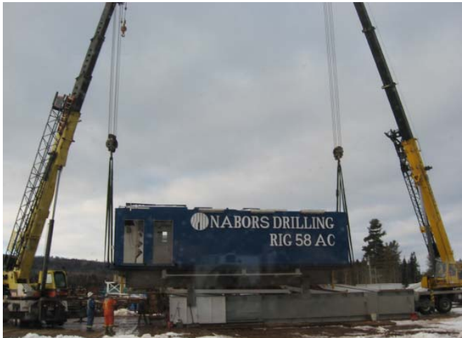
Pinning the Nabors Rig # 58 Dog House in place at the D-48 Well Pad.
