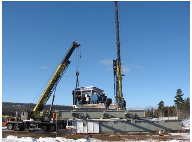
Positioning the Nabors Rig # 58 Drawworks in place at the D-48 Well Pad.
